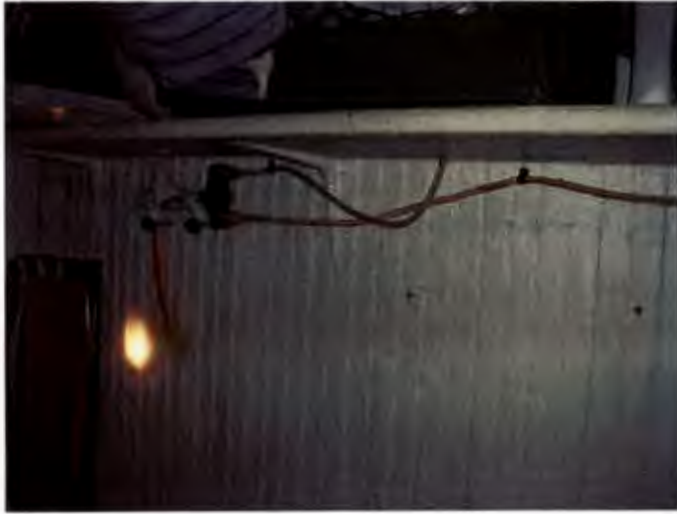
Over use of extension cords.
