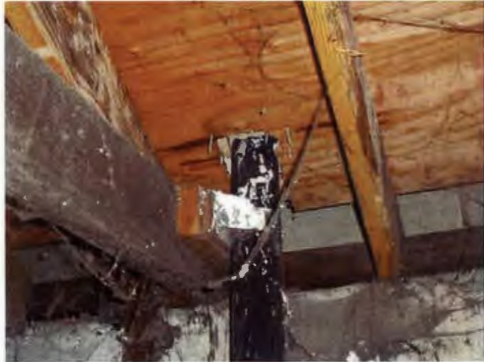
Visible signs of dry rot.
