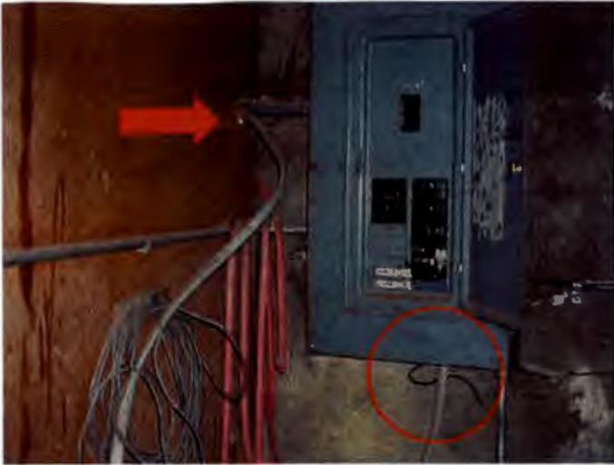
Wiring from electrical panel feeds 220 outlet
