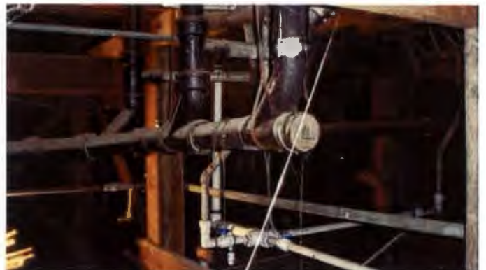
Plumbing cross connections and improper pipe material.
