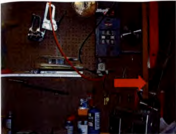
Unsecured 220 volt outlet; outlet wired from sub panel. Overuse of extension cords.
