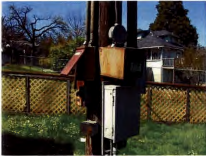
Open and insecure electrical boxes in concessions area.
