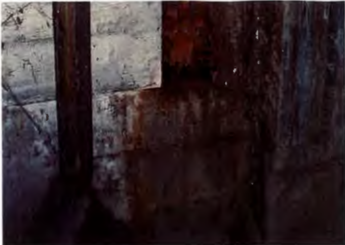
Roof downspout drains to grade along foundation. Visible signs of dry rot.
