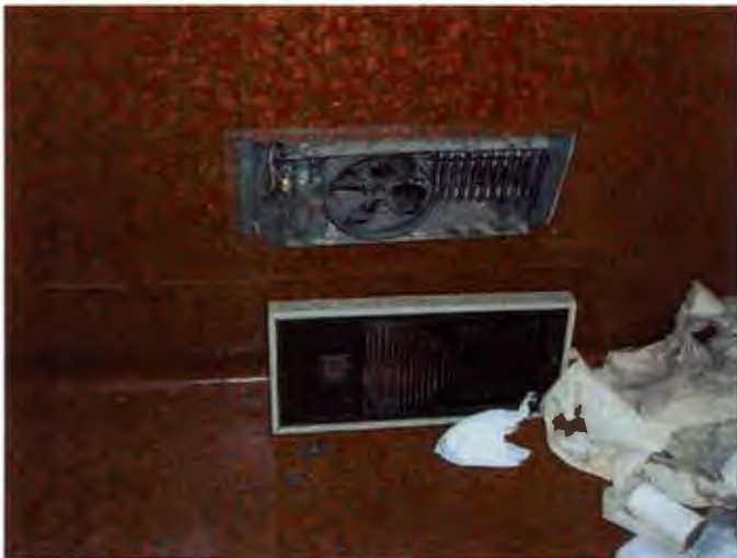
Unattached heater cover.
