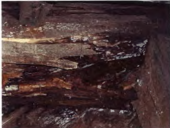
Visible signs of dry rot.
