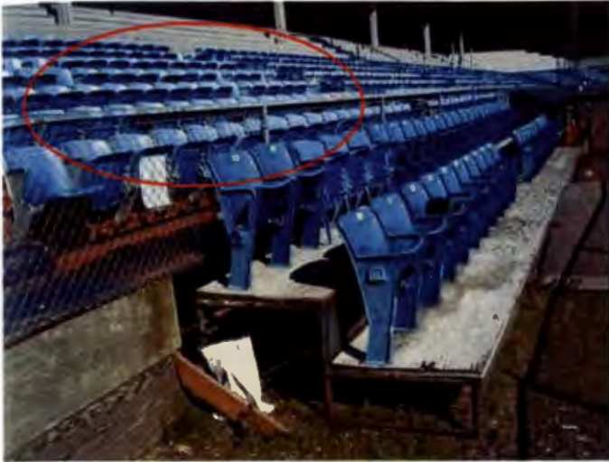
Structural support of metal bleacher seats corroded.
