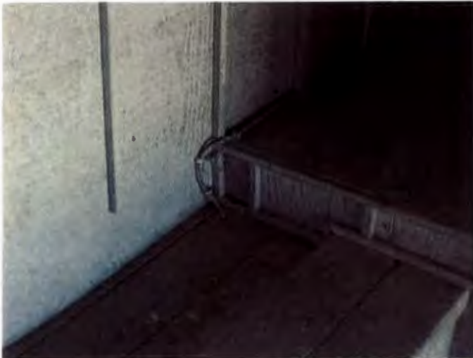
Unprotected wiring in wooden bleacher section.
