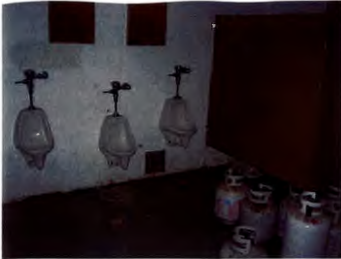
Urinals installed without venting; old toilet fixtures not properly sealed.
