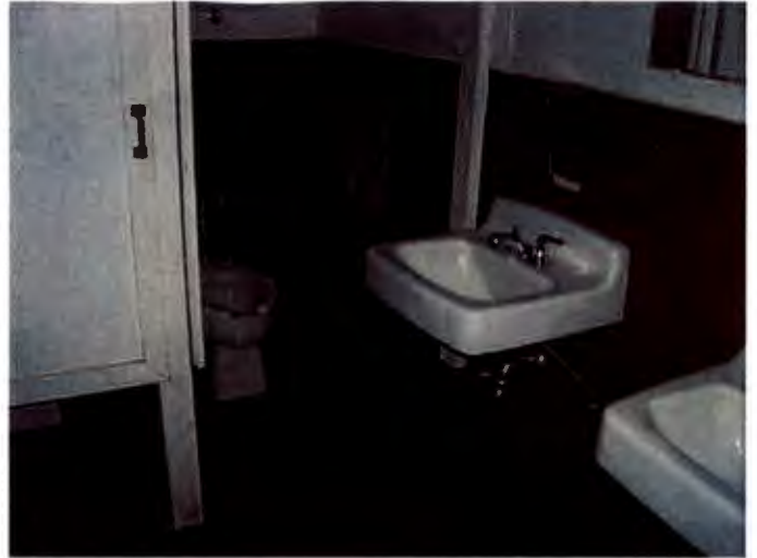
Lavatory sink projects into toilet stall.
