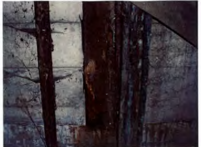
Roof downspout drains to grade along foundation. Visible signs of dry rot.
