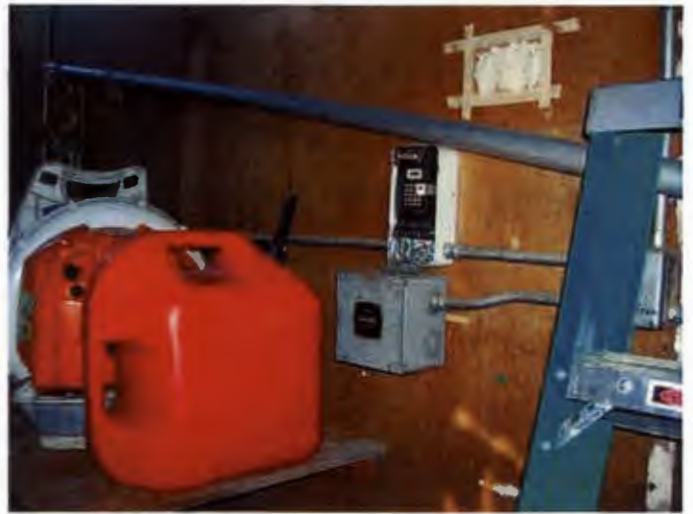
Irrigation control box missing cover, fumes from gas can be source of possible ignition.
