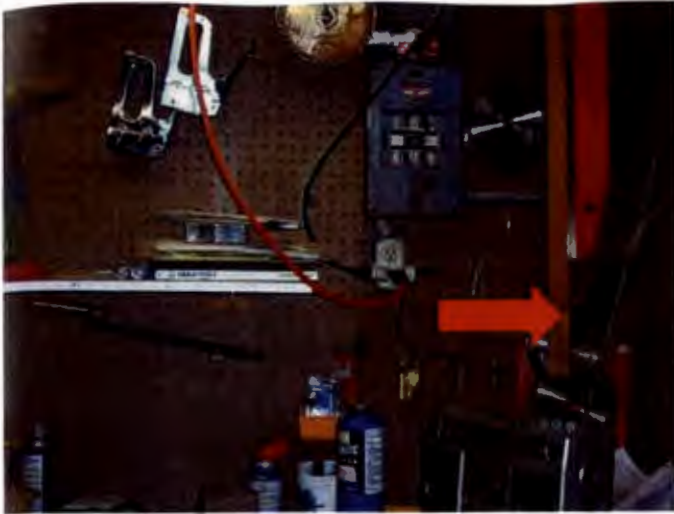
Unsecured 220 volt outlet; outlet wired from sub panel. Overuse of extension cords.
