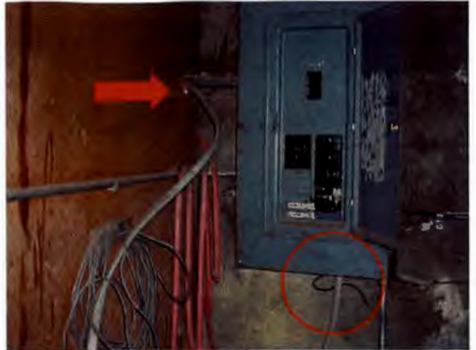
Wiring from electrical panel feeds 220 outlet
