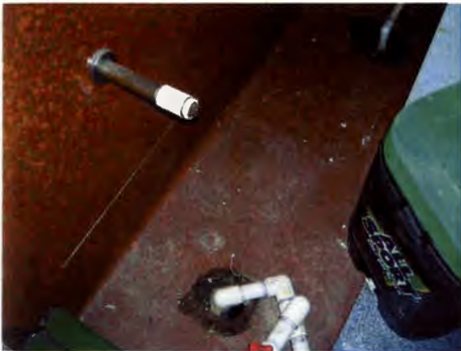
Open unvented drains to sanitary sewer system; source of sewer and sewer gas and access point for rats and vermin.
