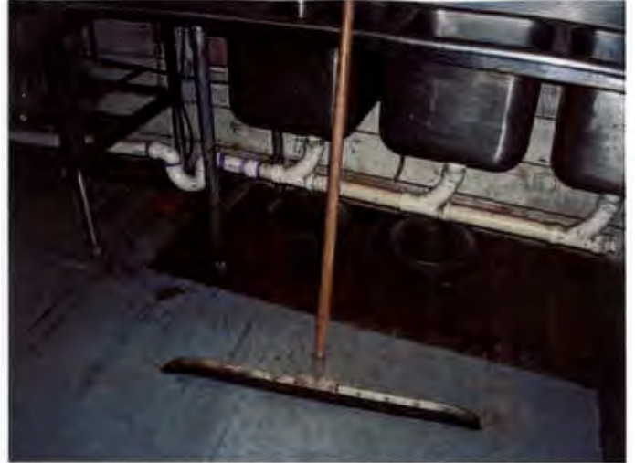
Leaky plumbing under sink drains.
