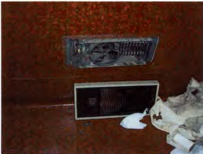
Unattached heater cover.
