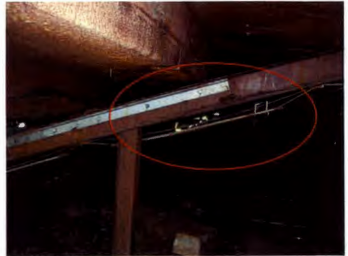
Electrical conduit corroded and broken, suspended with electrical wiring.
