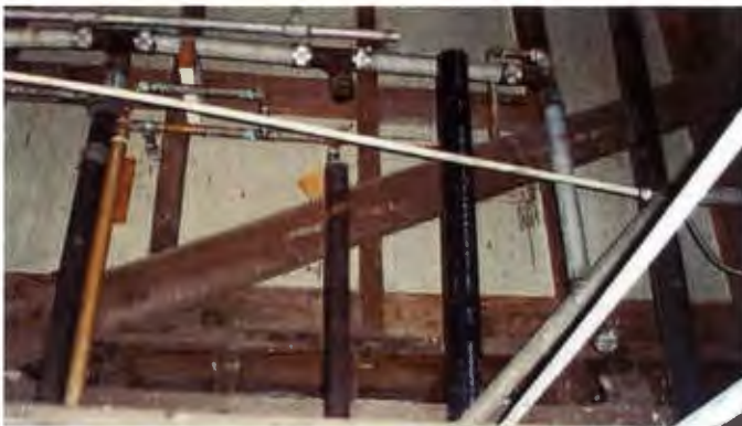
Plumbing cross connections and improper pipe material.
