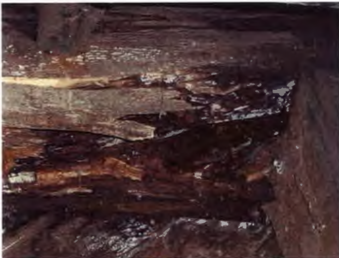
Visible signs of dry rot.
