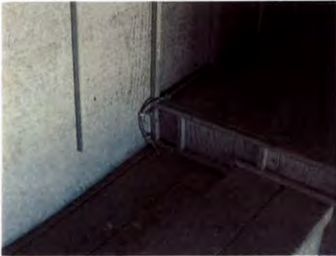
Unprotected wiring in wooden bleacher section.
