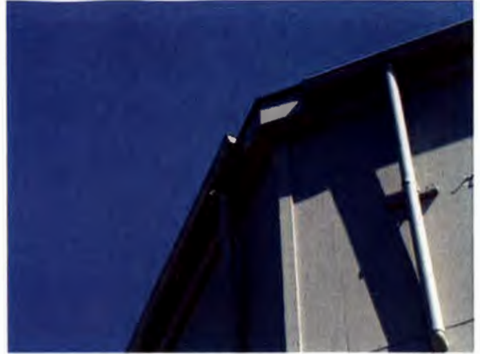
Downspout(s) disconnected from gutter. Gutters are not supported along roof edge.
