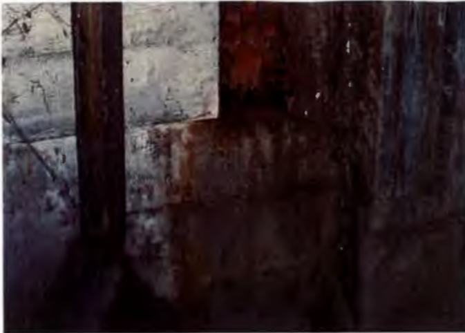
Roof downspout drains to grade along foundation. Visible signs of dry rot.
