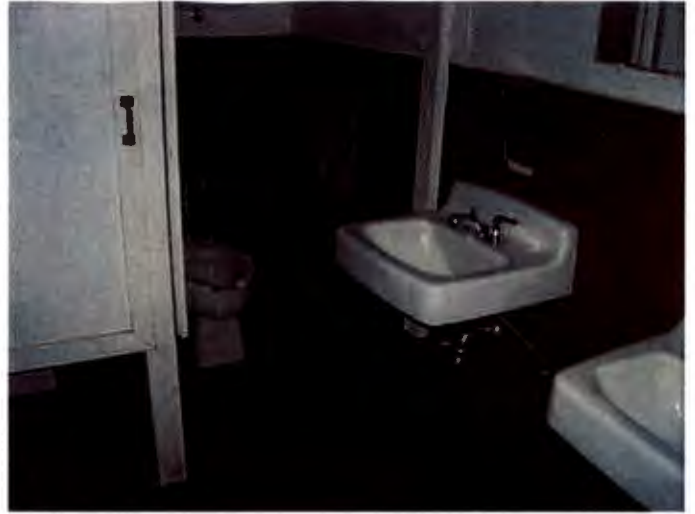
Lavatory sink projects into toilet stall.
