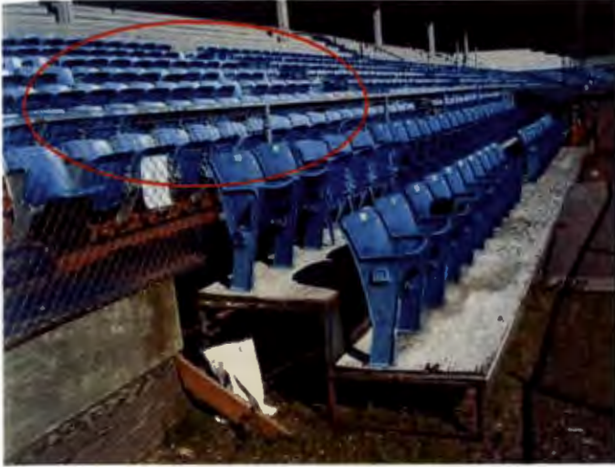
Structural support of metal bleacher seats corroded.
