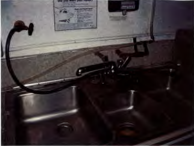
Non-compliant plumbing and garden hose in food prep area.
