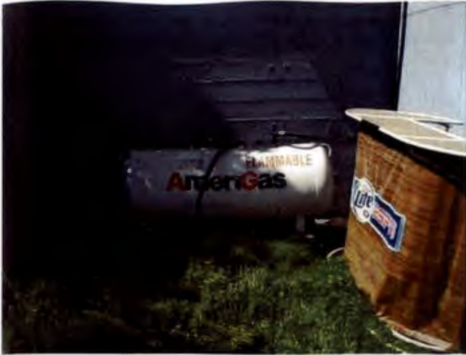
Propane accessible and open to the public.
