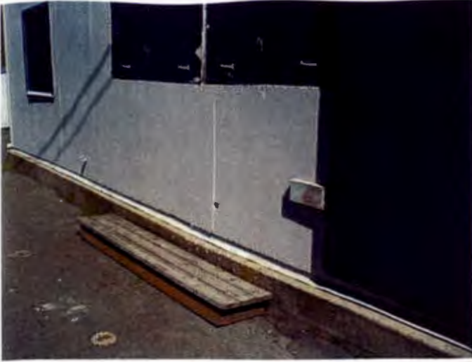
Temporary, non-secured steps to concession stand.
