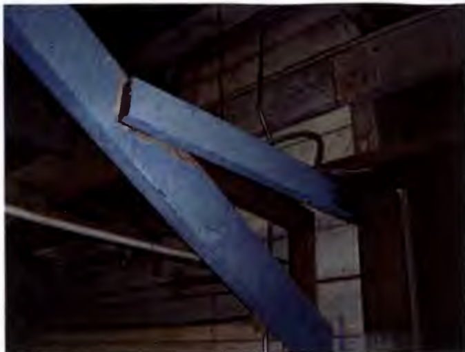
Alteration to structural framing.
