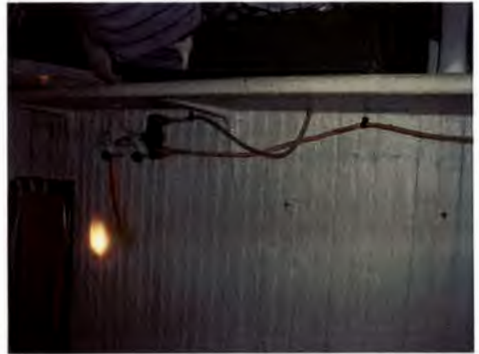
Over use of extension cords.
