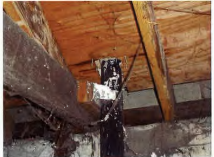
Visible signs of dry rot.
