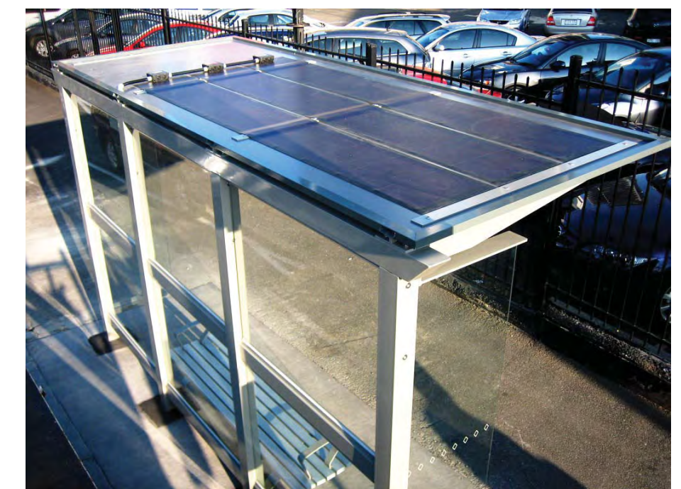
Energy Conservation -Solar Panels on Bus Stop
