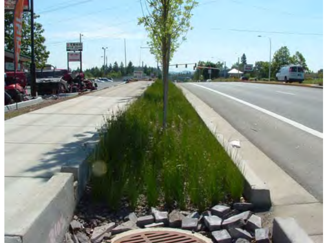
Flow-through planters serve for both landscaping and bioretention.
