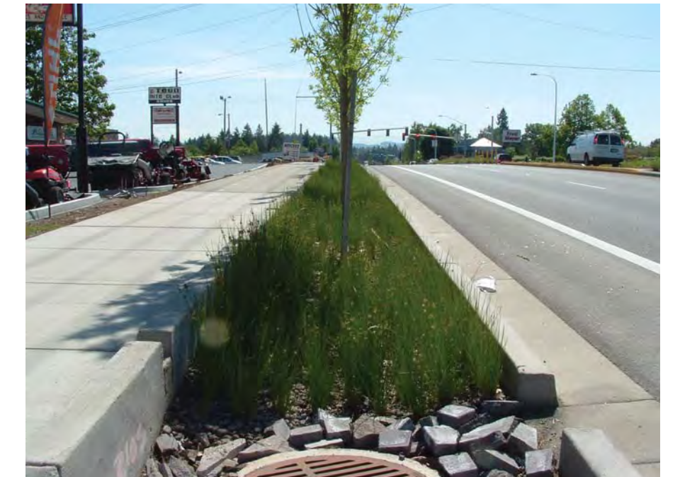
Stormwater Treatment -Flow Through Planter
