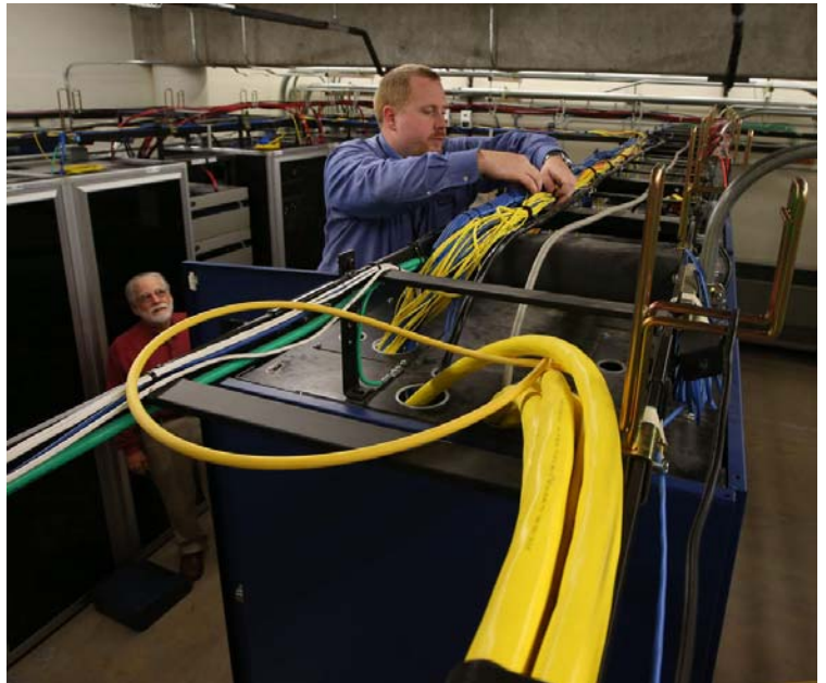
An ISP connects the fiber to a rack in the WIX.
