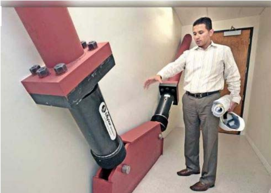
City of Santa Clarita Senior Engineer Mike Hennawy discusses the fluid viscous damper system that works as a shock absorber fitted to one of eight two story structural steel braces that have been added to support Santa Clarita Hall building in Valencia as part of an earthquake retrofit project. Signal photo by Dan Watson.
