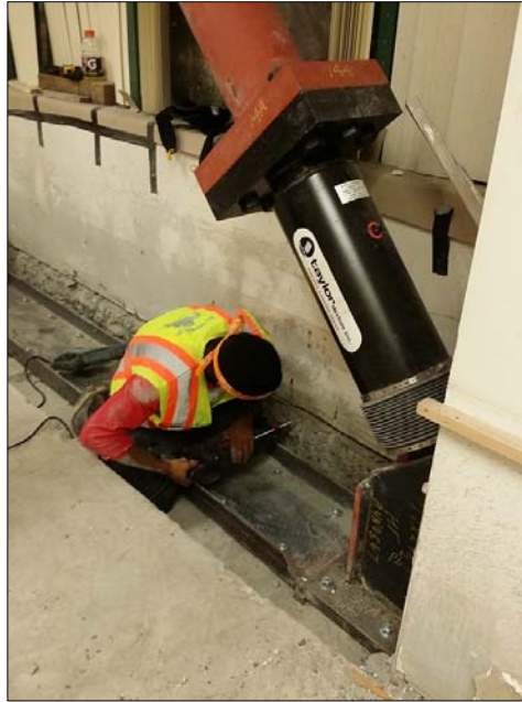
A typical damper shown above weighs about 600 lbs and is about 4' long with a 10" diameter. The damper is attached to a steel pipe with 3" thick steel plates.
