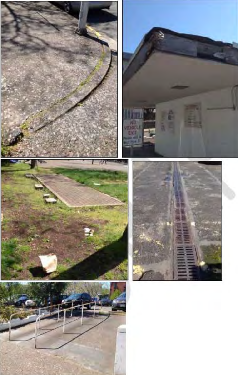
Photos: Top left: image of access ramp damage; top right: image showing example of damage to building; middle left: image shows green space on property with utility boxes and garbage; middle right: deterioration of pavement shown with holes and uneven surface; bottom: access ram shown.
