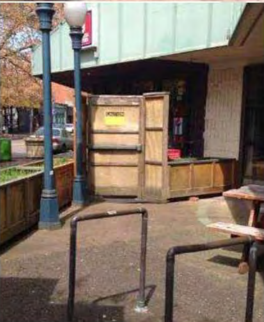
Photo: Top: image shows building deterioration; middle left: image shows south outside seating area, middle right: shows damage to planter in south outside seating area; bottom: shows exit door for south outside seating area.
