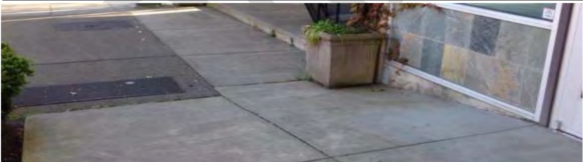
Photo: Top: view of property from Pearl Street; bottom photo shows ramp with questionable angle for accessibility.
