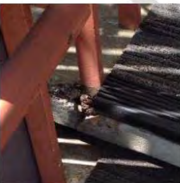
Photos: Top: View of property from West 8 th Avenue and West Park Street; middle left: image shows example of cracks in pavement on sidewalk outside building; middle right: image shows wear; bottom: image shows damage in cement at base of stair railing.
