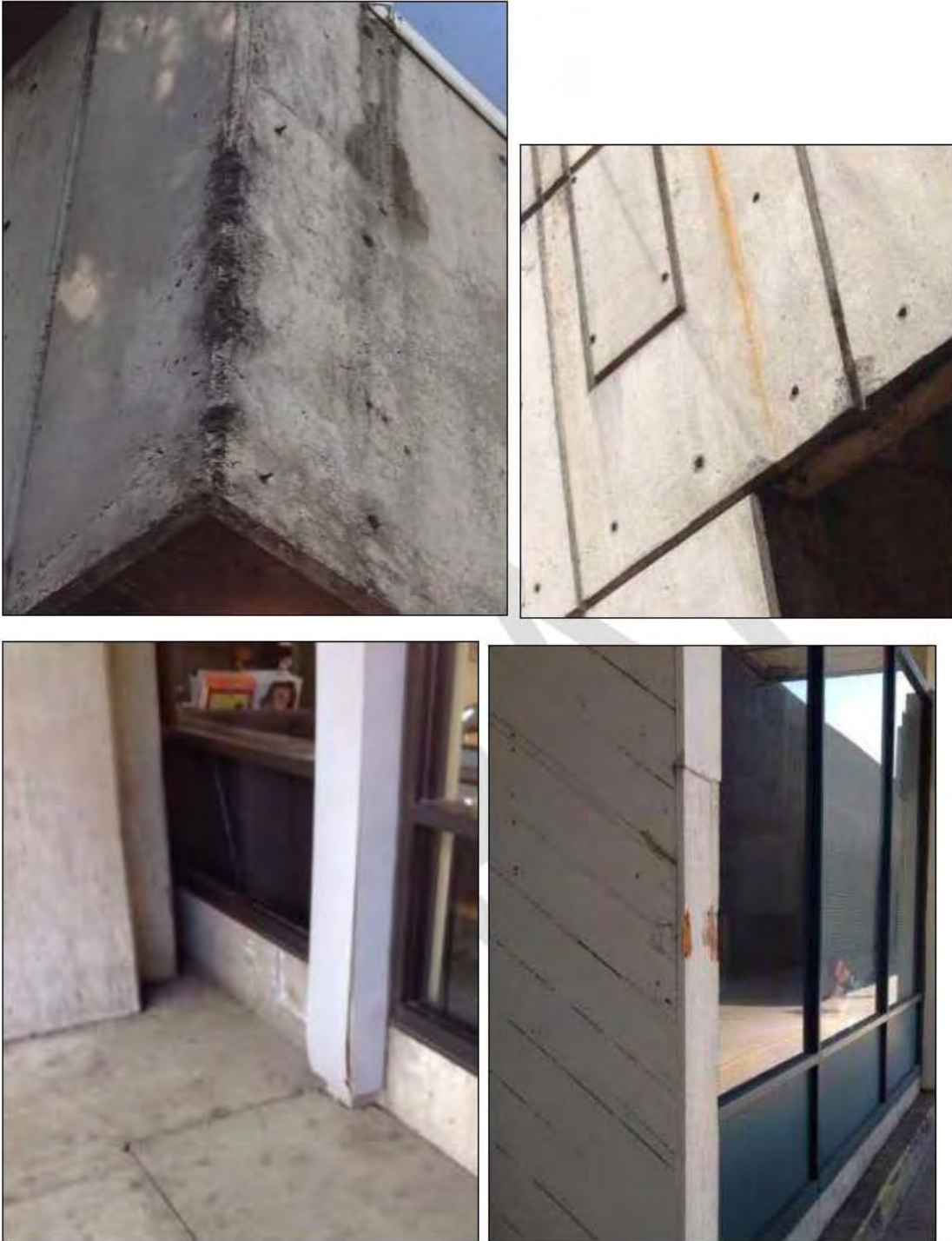
Photo: Top: examples of damage on exterior of structure; bottom: images showing examples of façade damage.
