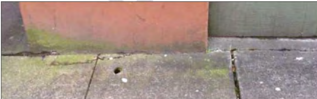
Photo: Top left: view of property from East Broadway; top right: image shows example of façade wear; bottom: cracks in pavement at base of building.
