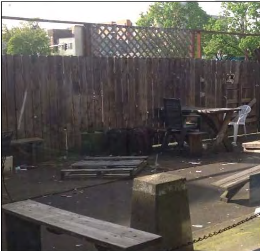
Photo: Top: view of property from Olive Street; bottom: view of back patio damage.
