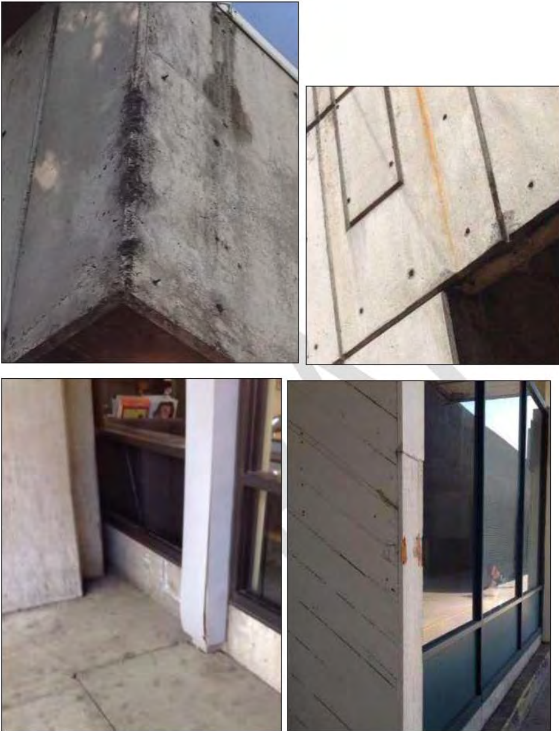
Photo: Top: examples of damage on exterior of structure; bottom: images showing examples of façade damage.
