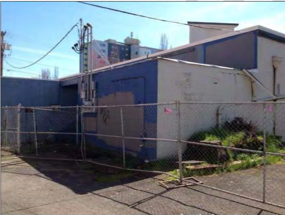
Photo: top and bottom images show back side of building with damage, broken fencing, deteriorated building, overgrown vegetation, graffiti and damaged pavement.
