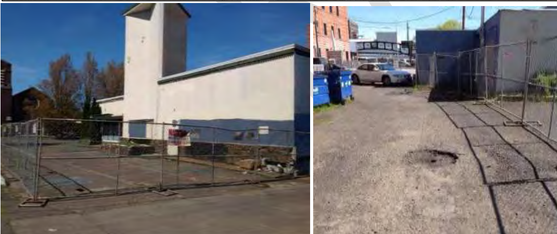
Photo: Top: shows property from SW corner of 11 th Ave and Charnelton St, Library can be seen in background; bottom left: shows property from se corner; bottom right: damage to pavement that provides access to parking area behind building.
