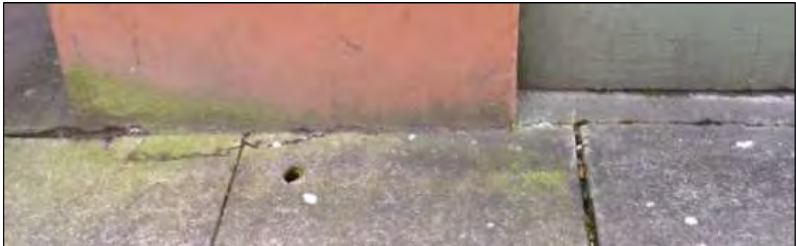
Photo: Top left: view of property from East Broadway; top right: image shows example of façade wear; bottom: cracks in pavement at base of building.
