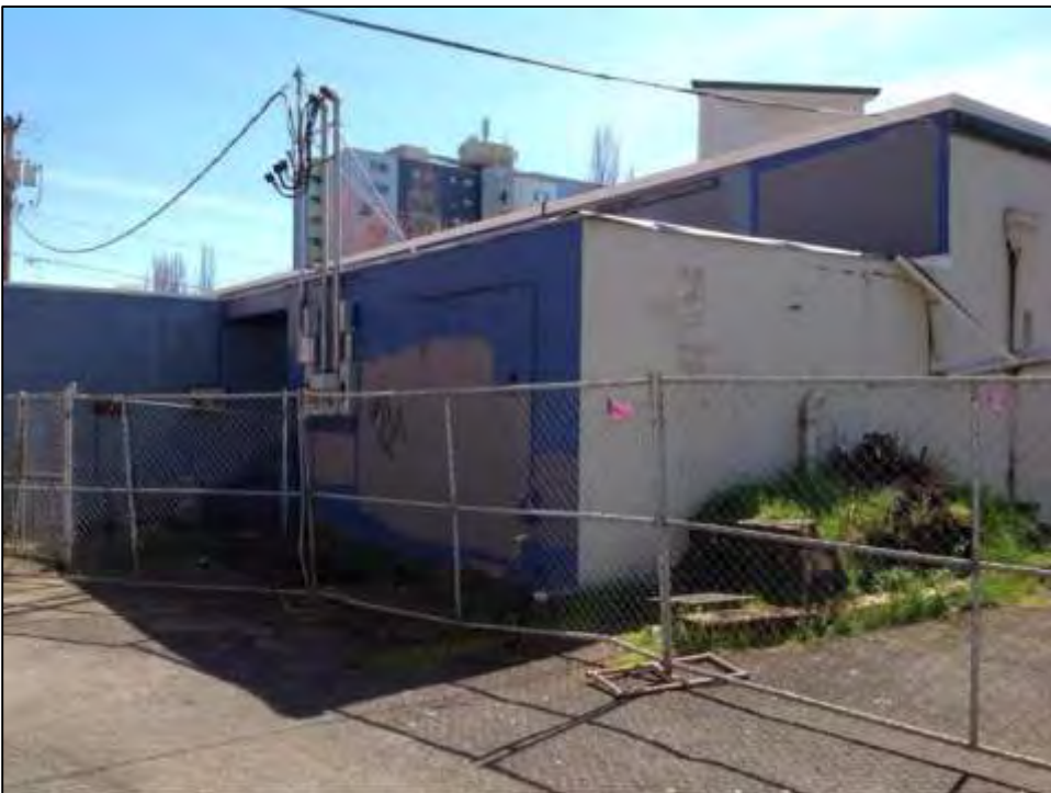
Photo: top and bottom images show back side of building with damage, broken fencing, deteriorated building, overgrown vegetation, graffiti and damaged pavement.
