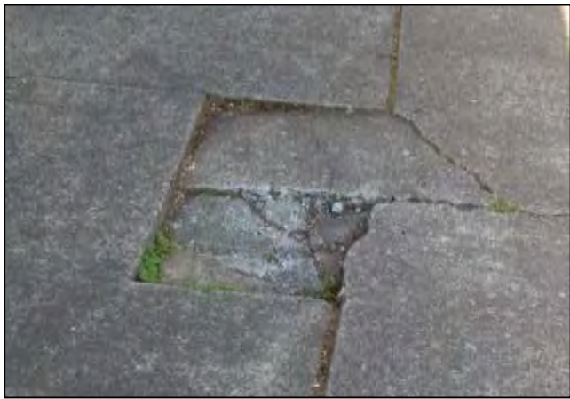
Photo: Top: front of building facing Willamette Street; bottom: damage in pavement in back of building.
