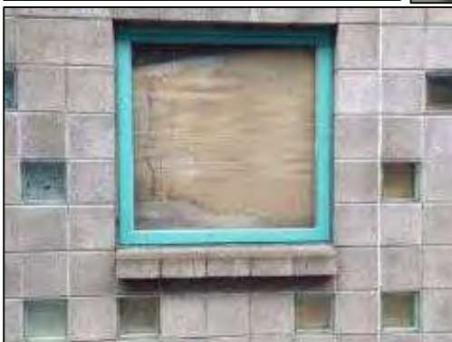
Photo: Top: view of property from Olive Street; middle left: cracks visible on structure; middle right: image shows an example of white material in cracks in structure; bottom: image shows example of window with water damage inside.
