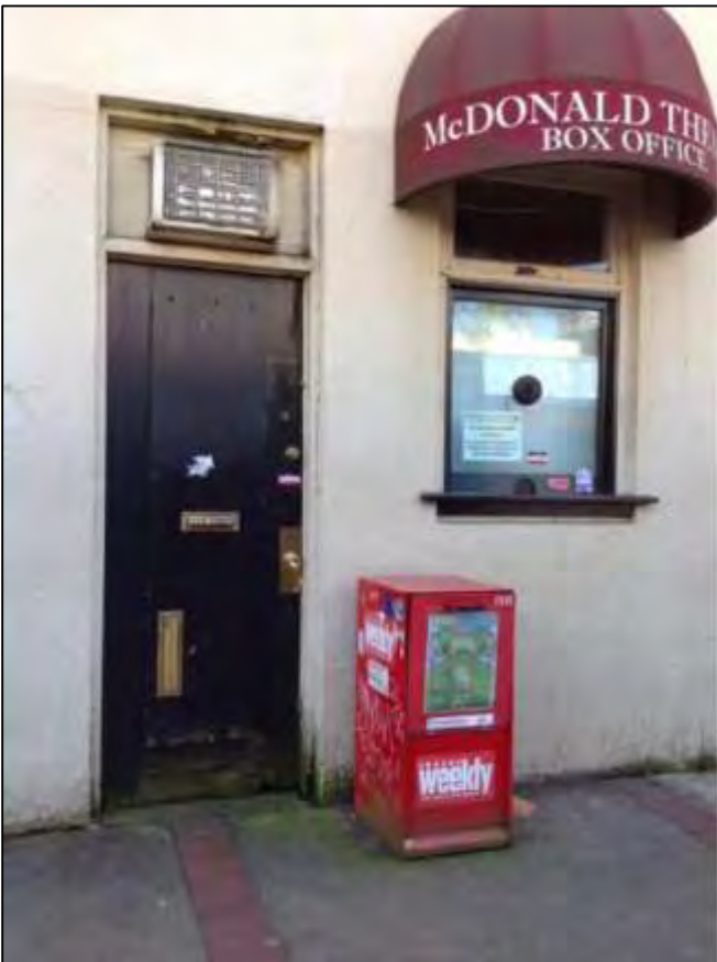
Photo: Top: View of property from West 10 th Avenue and Willamette Street; bottom: shows example of damage on building, especially where the door meets the sidewalk
