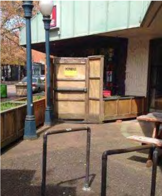
Photo: Top: image shows building deterioration; middle left: image shows south outside seating area, middle right: shows damage to planter in south outside seating area; bottom: shows exit door for south outside seating area.
