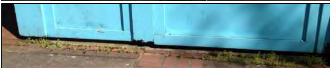
Photo: Top: view of property west side from Olive Street; middle left: photo is east side of building from service court; middle right: detail photo of entryway off Olive Street; bottom: example of wood damage on exterior.
