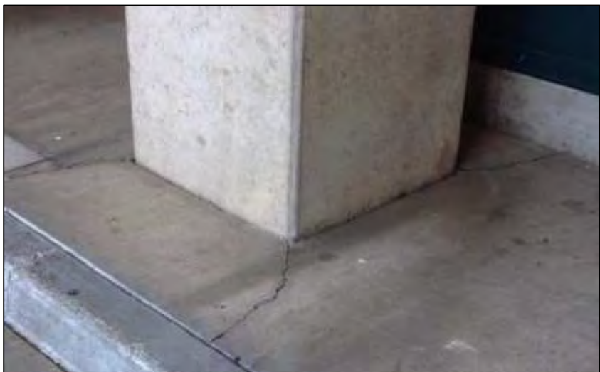
Photo: Top left: image shows broken sign; top right: large open space; bottom: image shows cracks at base of pillar.
