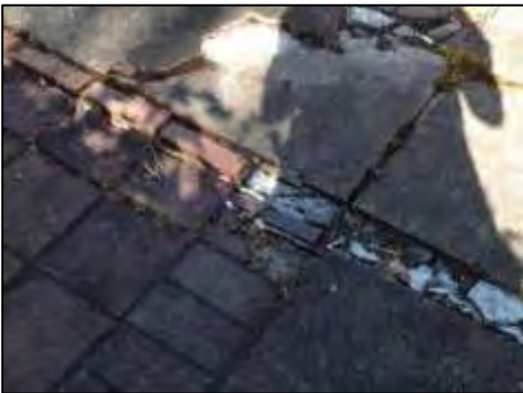
Photo: Top: image shows cracked cement along railing; middle: large open space; bottom: example of broken walkway.
