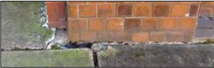
Photo: Top: view of property from East 10 th Avenue and Willamette Street; bottom: image shows damage at base of building.
