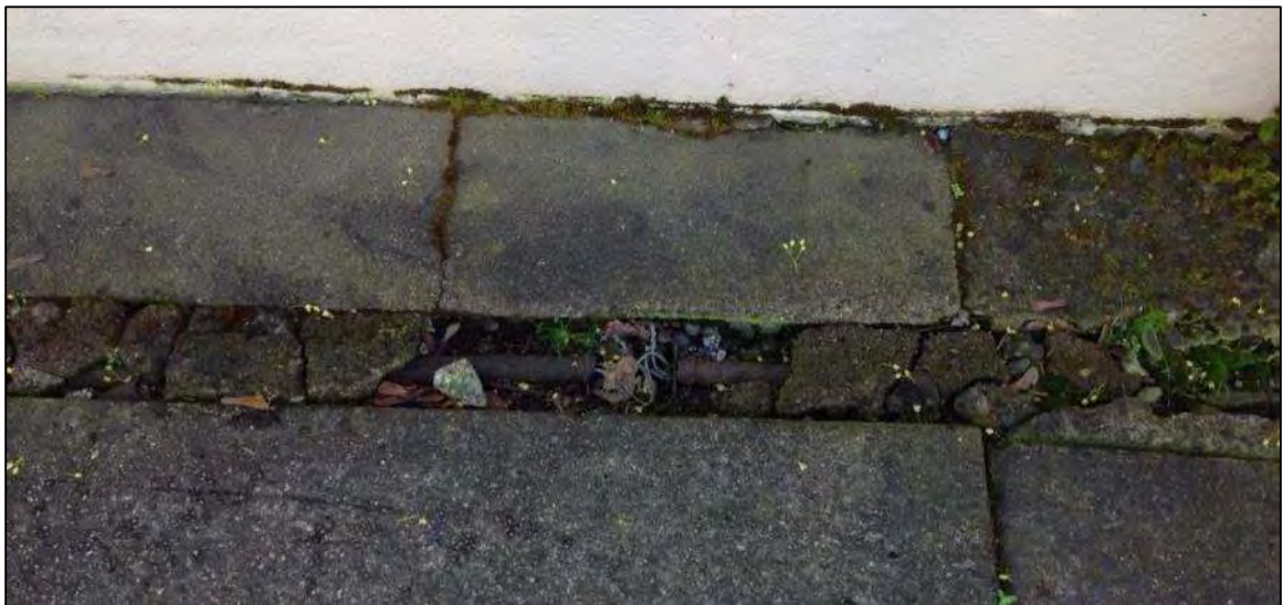
Photo: bottom image shows wiring in an exposed underground pipe.
