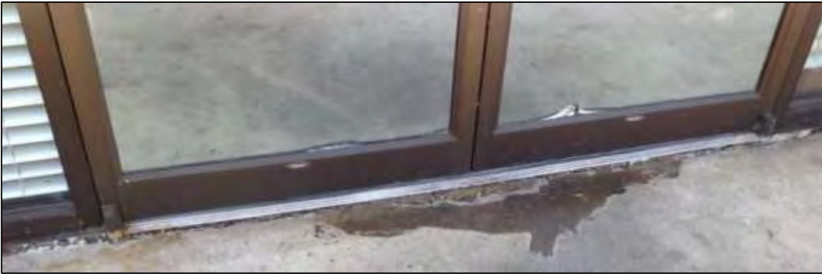
Photo: Top left shows where sign was partially removed; top right: damaged exterior brick work; bottom: damaged entryway.
