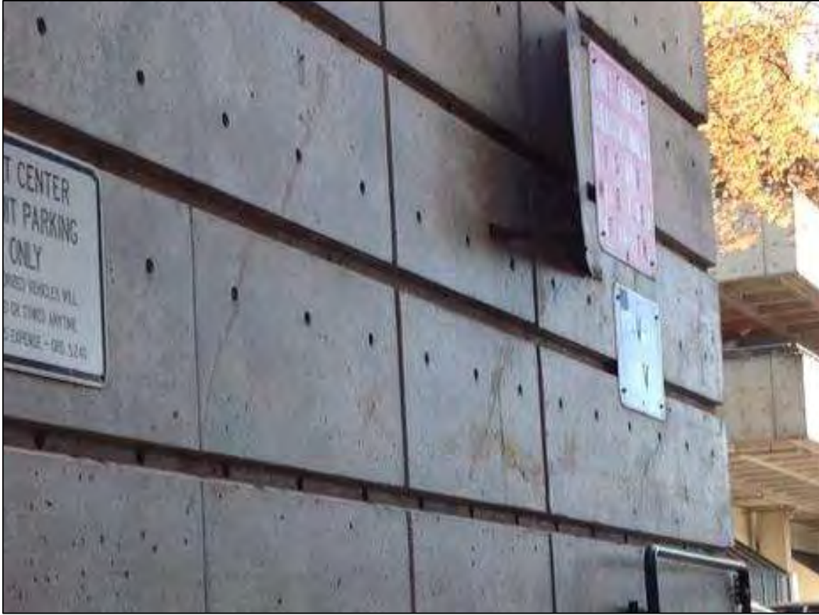
Photo: Image shows example of cracks along surface (diagonal lines).
