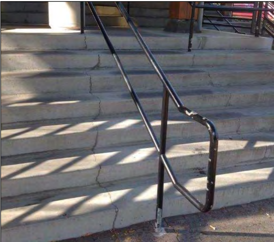
Photo: top left: image shows damage to pipe on rear of building; top right: picture shows an example of sidewalk width; bottom: image shows cracks in steps
