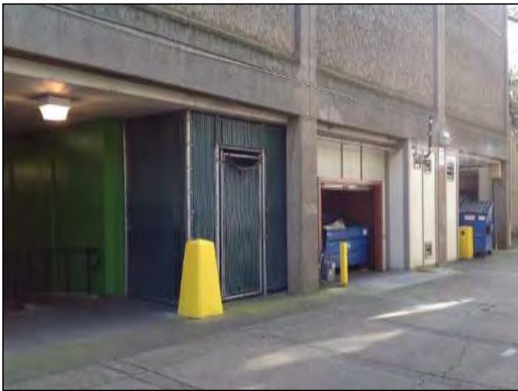
Photo: Top: example of building condition in interior pathways; bottom: view of alley and area of access to pedestrian walkway to restroom.
