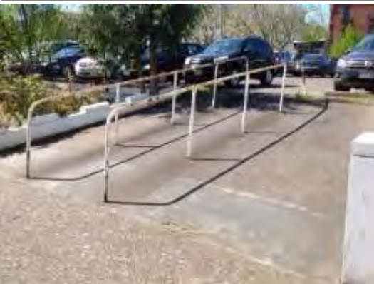
Photos: Top left: image of access ramp damage; top right: image showing example of damage to building; middle left: image shows green space on property with utility boxes and garbage; middle right: deterioration of pavement shown with holes and uneven surface; bottom: access ram shown.
