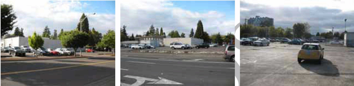
Map ID# 165 through 167 —Tax lots 2200, 2300, and 2400 of Map 17033142 (Peace Health surface parking—East): Single-story structure on tax lot 2400 is vacant, with cracks in wall, exposed boards, broken foundation. Improvement to land ratio: .09, .09 and .05; Building rating: –
