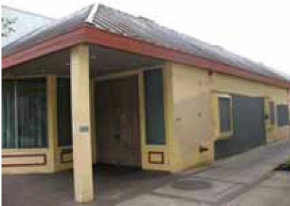
Map ID# 93 —Tax lot 3400 of Map 17033113 (vacant former gallery): Appears vacant. Single-story building with oxidizing roof, peeling exterior wall paint and substantial graffiti. Improvement to land ratio: 1.75; Building rating: ±
