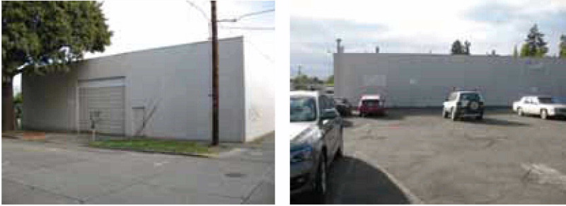
Map ID# 164 —Tax lot 2100 of Map 17033142 (Peace Health storage): Single-story building is used for storage. Cracks in wall, paint and stucco peeling, graffiti. Improvement to land ratio: .65; Building rating: ±
