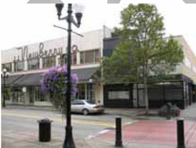
Map ID# 20 —Tax lot 1700, Map 17033113 (Downtown Athletic Club - Newberry Childcare and offices): Old J.J. Newberry Co. building. Rust stains from tie-rods along the side of the building, eroding brick work, and peeling paint. EWEB notes that steam conversion is needed. Improvement to land ratio: .3.2; Building rating: ±
