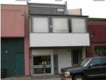
Map ID# 99 —Tax lot 4700 of Map 17033113 (860 Olive St.): Vacant ground floor. Wood siding needs repair, paint peeling in places. Improvement to land ratio: 8.43; Building rating: ±
