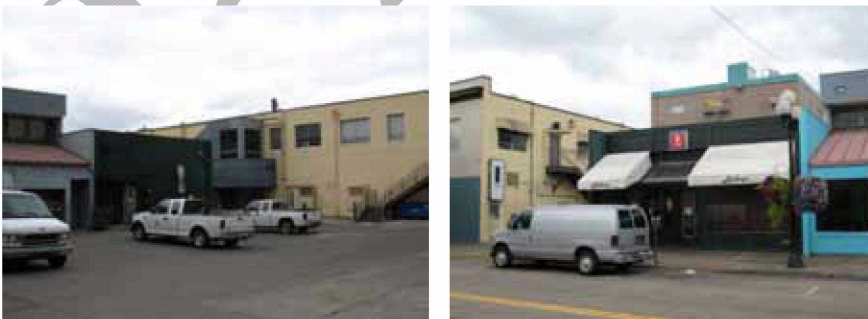
Map ID# 64 —Tax lot 2800 of Map 17033113 (Luckey’s): Single-story building. Awnings (glass and fabric) need cleaning, sealing and repair; window frames peeling and deteriorating. Improvement to land ratio: 2.09; Building rating: ±
