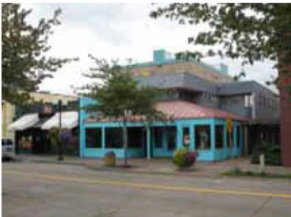
Map ID# 63 —Tax lot 2700 of Map 17033113 (Imagine Hair Salon): Building in need of maintenance (paint peeling, siding pulling off in places). Improvement to land ratio: 3.6; Building rating: ±
