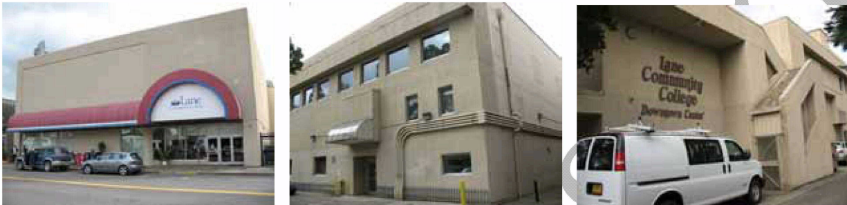
Map ID# 6 —Tax lot 12800 of Map 17033114 (Lane Community College Downtown Center): Building shows some wear and lack of maintenance (peeling exterior, graffiti) LCC has announced plans to build a new downtown center and to vacate this building. Upper floors have very few windows. Improvement to land ratio: 8.3; Building rating: ±
