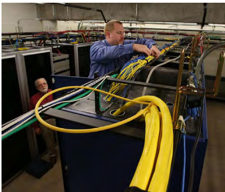
An ISP connects the fiber to a rack in the WIX.
