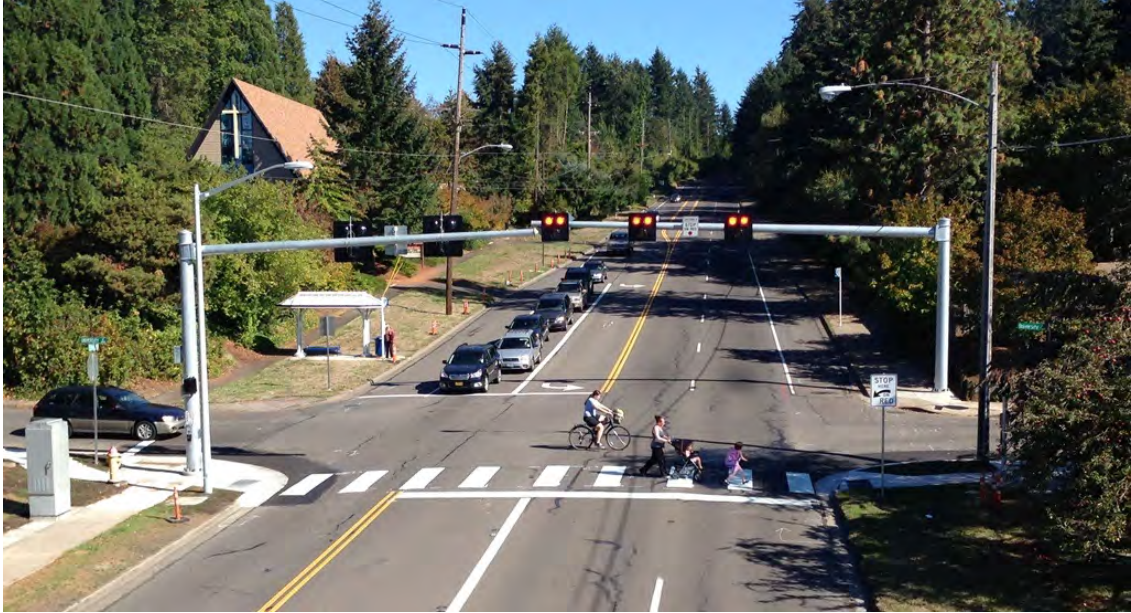
Pedestrian Hybrid Beacon on 30th Avenue
