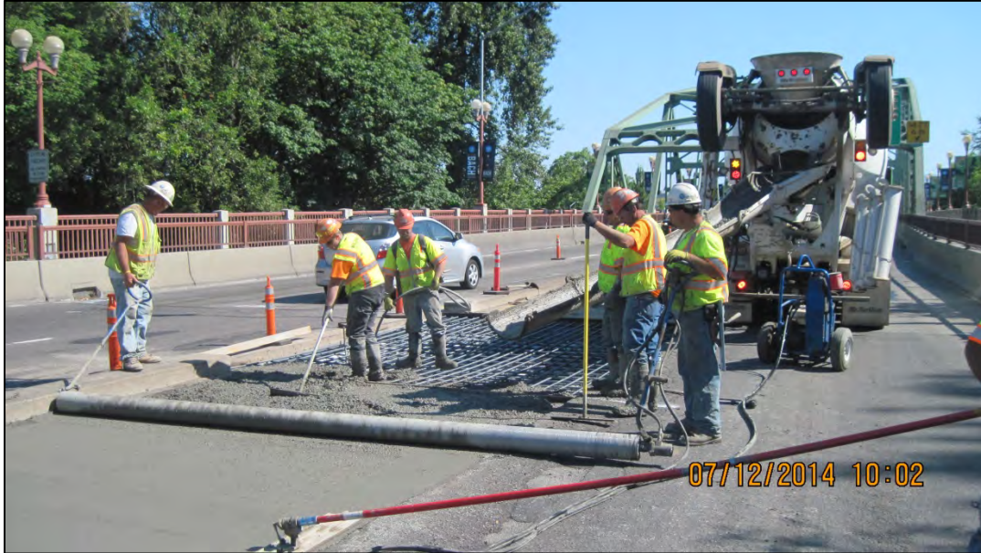
Portland cement concrete overlay paving on Coburg Road between the viaduct and Ferry Street Bridge
