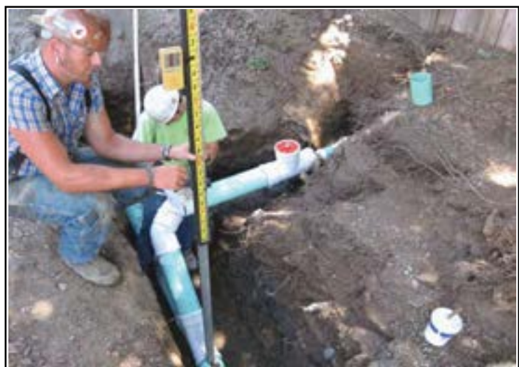
Service line being built at the property line as part of the Community Wastewater Sewers project.
