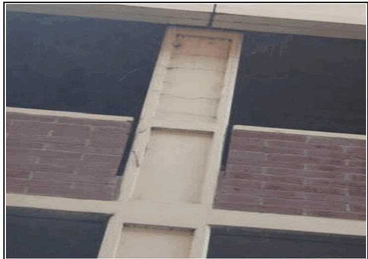
Pearl Street Garage - Spall in Column.
