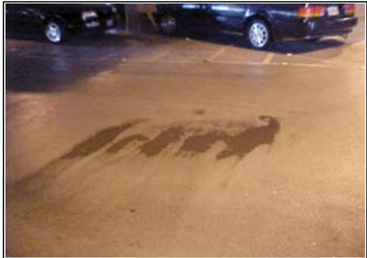
Example of wear on Overpark deck.
