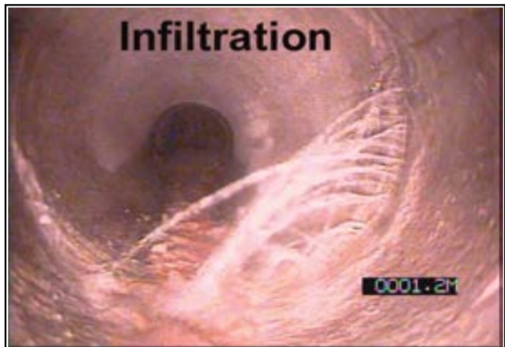
Wastewater pipe with groundwater leaking into the system.
