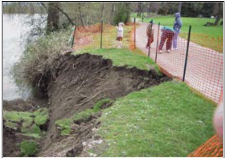
Skinner Butte Park river bank failure March 2012
