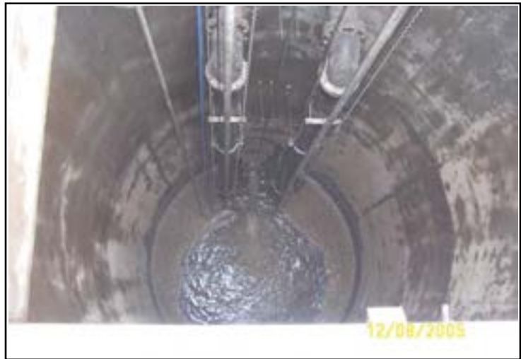
The inside of pump stations consist of wet wells (shown here) to store flows before they are pumped further in the system and dry wells for the mechanical elements. Replacing worn-out pumps, electrical components or piping are some of the improvements made under the Pump Station Rehabilitation program.
