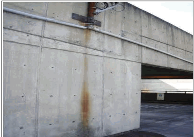
Water leak in wall of Parcade Garage.
