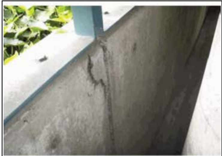
Hult Garage, showing spall in exterior wall
