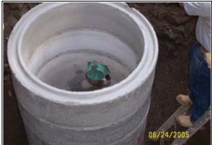
New manholes are one component of the infrastructure that gets built in conjunction with new development.
