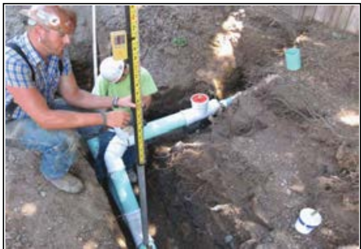
Service line being built at the property line as part of the Community Wastewater Sewers project.
