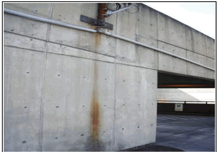
Water leak in wall of Parcade Garage.
