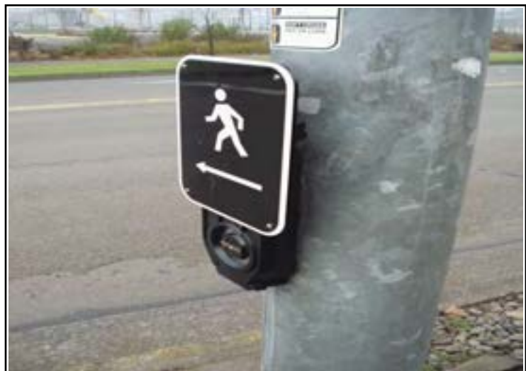
Audible Pedestrian Signal at 26th Avenue and Hilyard Street.
