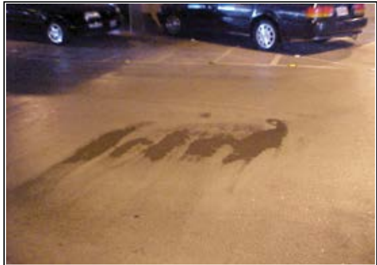
Example of wear on Overpark deck.
