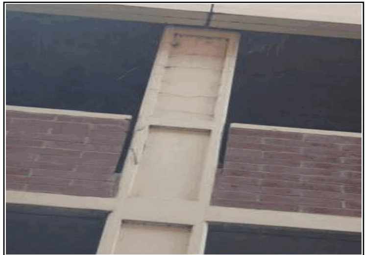
Pearl Street Garage - Spall in Column.
