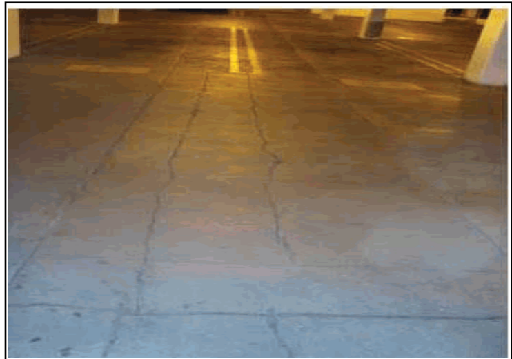
Broadway North Garage - Cracks in pour joint on level P1.
