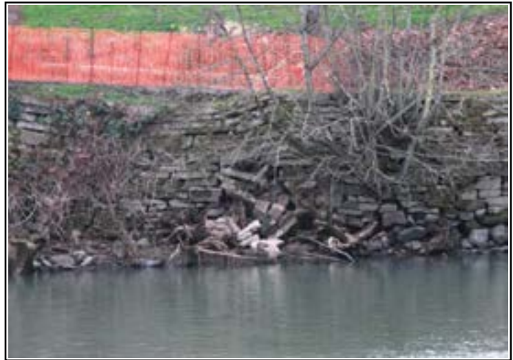
Failing concrete stacked retaining wall adjacent to the Owen Rose Garden.
