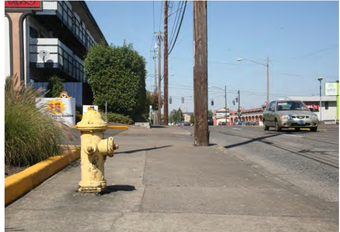
Example of utility conflicts in sidewalk.
