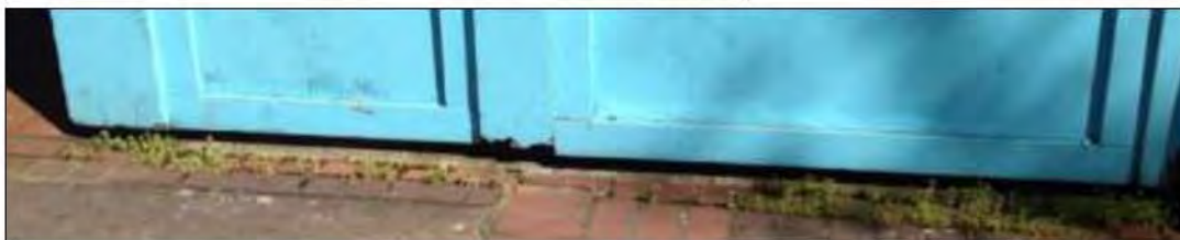
Photo: Top: view of property west side from Olive Street; middle left: photo is east side of building from service court; middle right: detail photo of entryway off Olive Street; bottom: example of wood damage on exterior.
