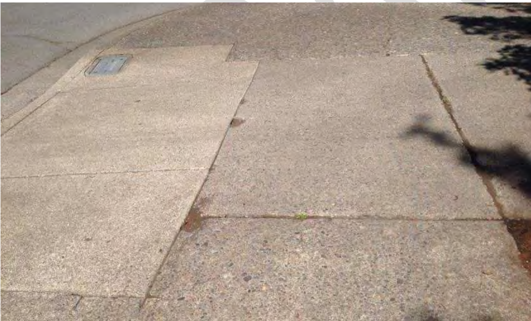
Photo: Top: view of property from Oak Street; bottom: image shows holes and cracks in pavement leading up to ramp
