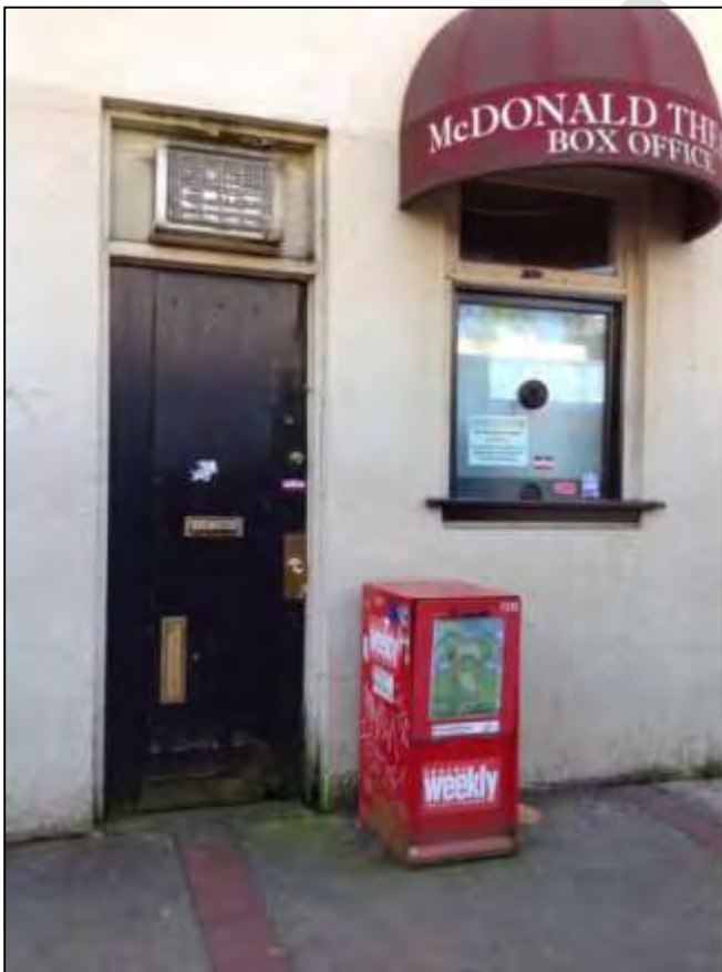
Photo: Top: View of property from West 10 th Avenue and Willamette Street; bottom: shows example of damage on building, especially where the door meets the sidewalk
