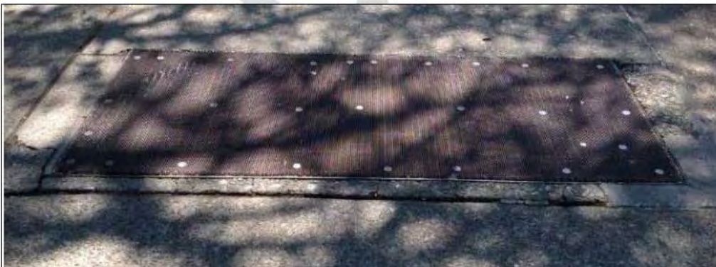
Photo: Top left: portable restroom on property, graffiti is covered by black box; top right: image shows plants growing on shelter; middle left: broken utility box; middle right: example of crooked bench; bottom: metal grate in damaged sidewalk
