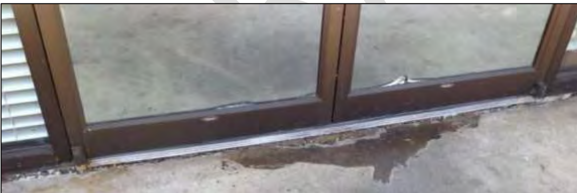
Photo: Top left shows where sign was partially removed; top right: damaged exterior brick work; bottom: damaged entryway.
