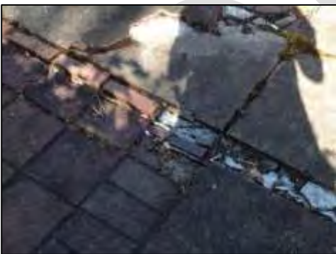
Photo: Top: image shows cracked cement along railing; middle: large open space; bottom: example of broken walkway.
