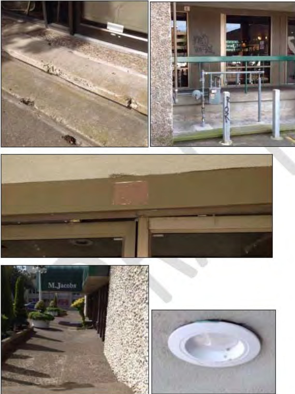
Photo: Top left: example of deteriorated cement; top right: property damage; middle: top of exterior door that is mis-aligned with structure; bottom left: entrance with concave entryway; bottom right: outside light fixture with wires exposed.
