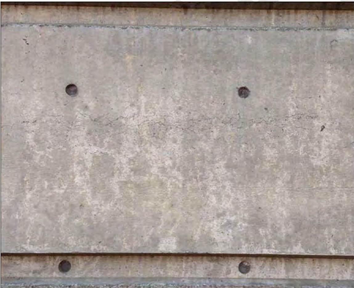
Photo: Top: image shows deterioration of steps; bottom: image shows cracks in cement of structure
