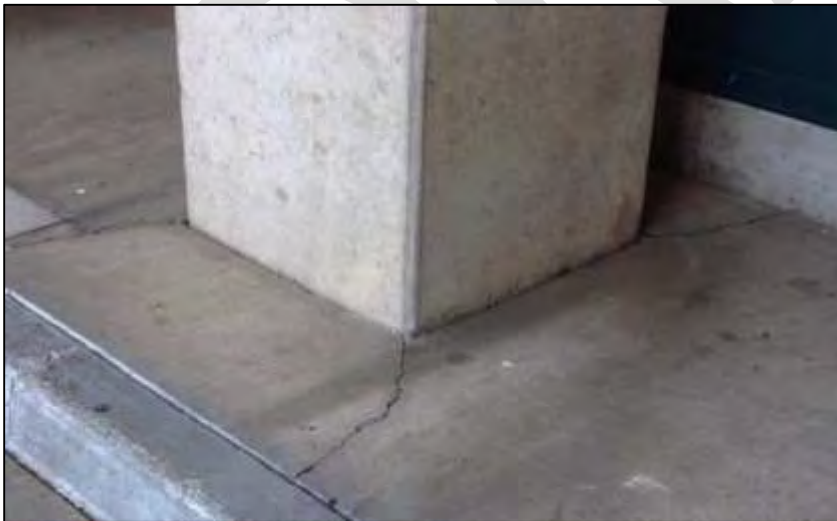
Photo: Top left: image shows broken sign; top right: large open space; bottom: image shows cracks at base of pillar.
