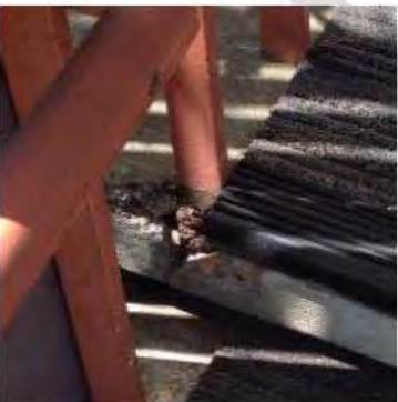
Photos: Top: View of property from West 8 th Avenue and West Park Street; middle left: image shows example of cracks in pavement on sidewalk outside building; middle right: image shows wear; bottom: image shows damage in cement at base of stair railing.
